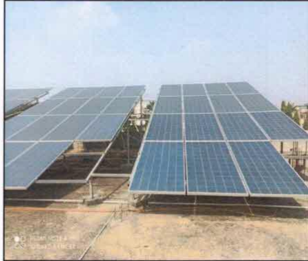
Photograph of Roof Top Solar PV Plant:
