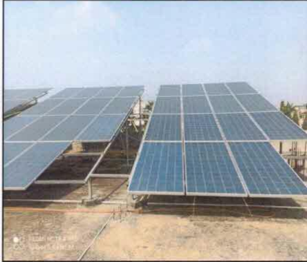
Photograph of Roof Top Solar PV Plant:
