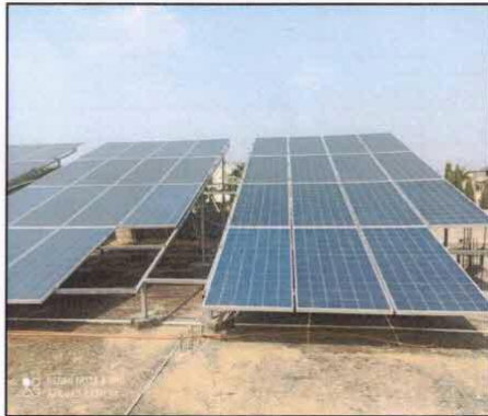
Photograph of Roof Top Solar PV Plant:
